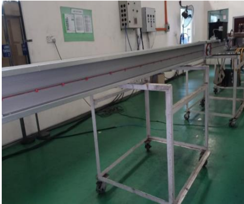
TMS – Temperature Monitoring System
